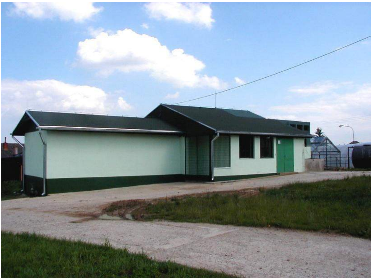
Figure 3. General view on the Biogas plant Kolíňany
